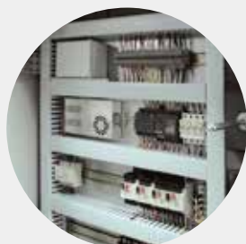
Intelligent Control Panel
